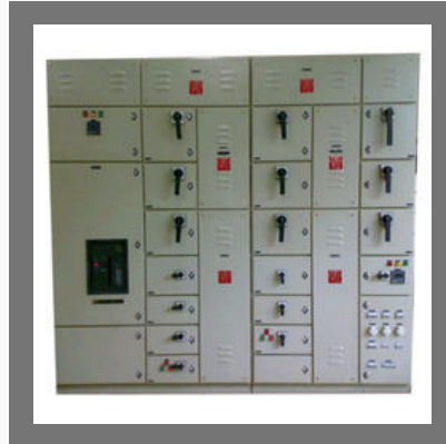
Distribution Control Panel
