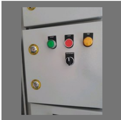
AC Drive Panel
