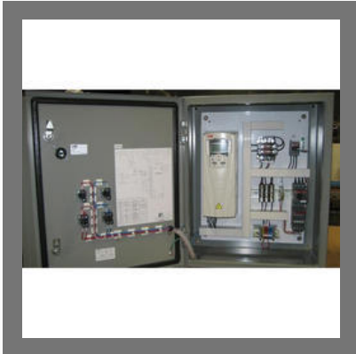
Single Phase VFD Panels
