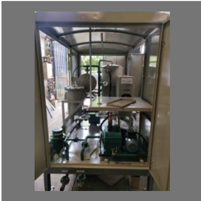
transformer oil filter machine
