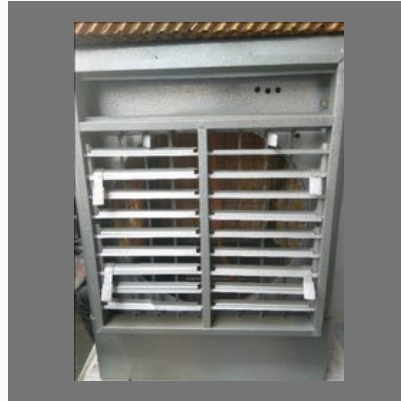
Big Tank Cooler
