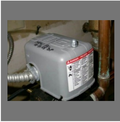
Water Pump Pressure Switch
