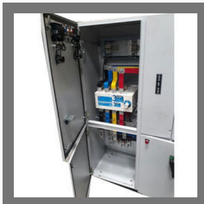
Power Control Panel
