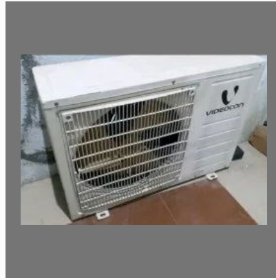
Air Conditioner Outdoor Unit
