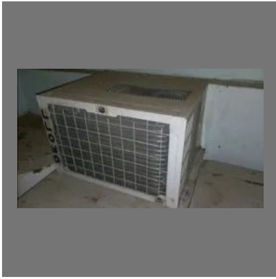
Air Conditioner Outdoor Unit
