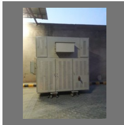
Kirloskar Dry Type Transformer, Installation And Shifting Along With Proper Servicing
