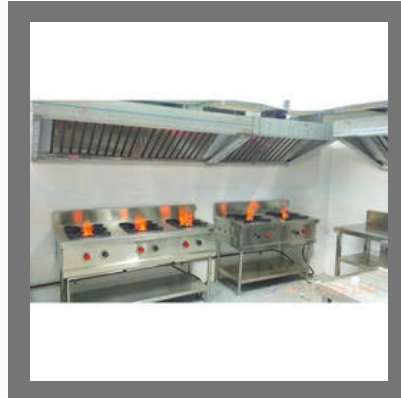
Commercial Kitchen Hood
