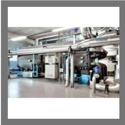
HVAC Fabrication Service
