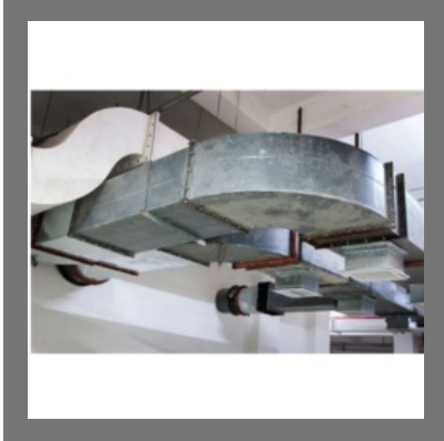
Air Conditioner Duct
