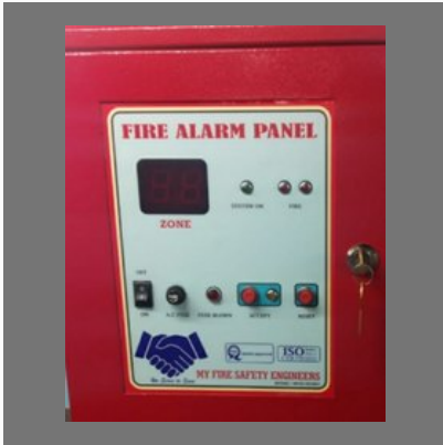
Conventional Fire Alarm Panel ( 4 core looping systems)
