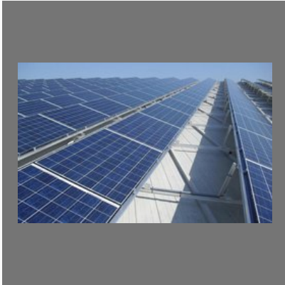
Industrial Solar Rooftop System
