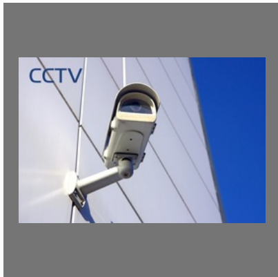
CCTV Camera Installation
