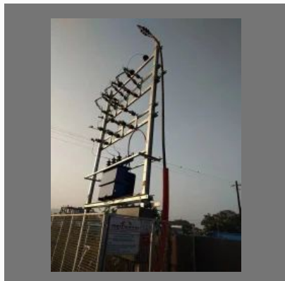
HT Installation Service
