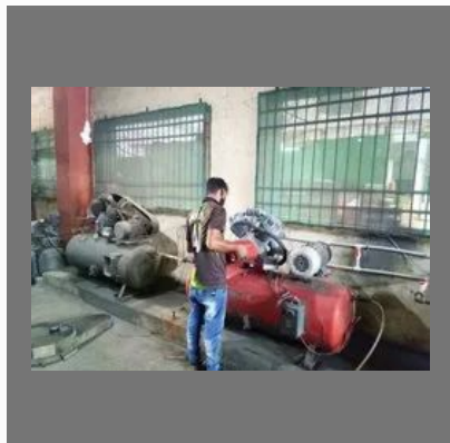
Air Compressor Maintenance Service
