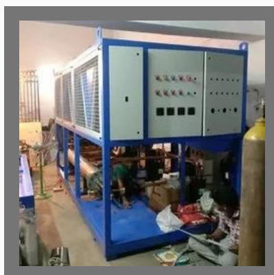
used industrial air cooled Chiller
