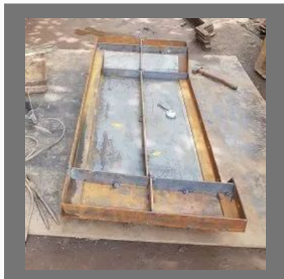
I Girder Shuttering Plate
