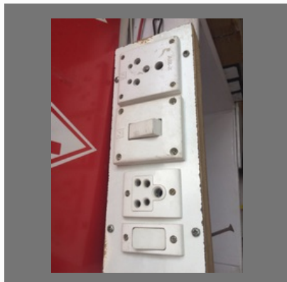
Electric Switch Board
