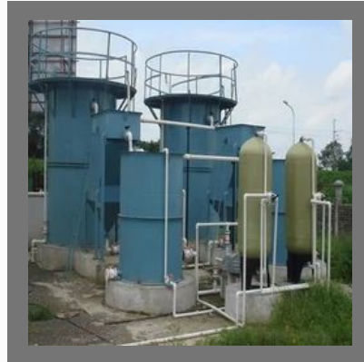
Containerized Effluent Treatment Plants
