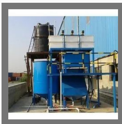
Sewage Treatment Plants
