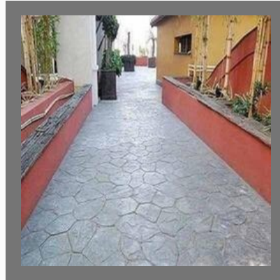
Stamped concrete Floor
