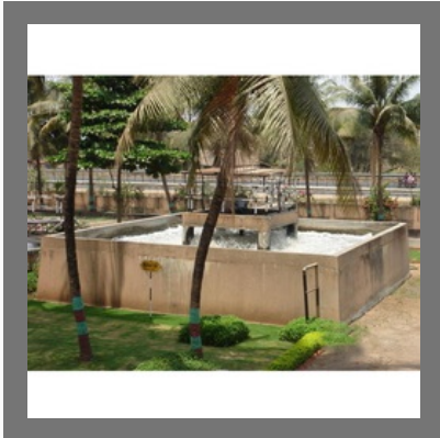
Waste Water Treatment Plant
