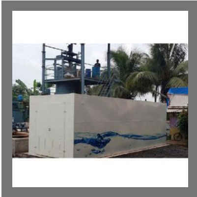
Containerized Sewage Treatment Plant
