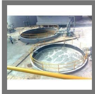
Effluent Treatment Plant
