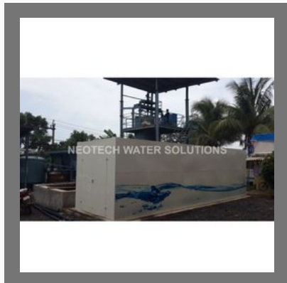
Packaged Sewage Treatment Plant
