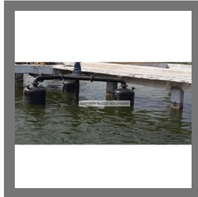
Floating Surface Aerator
