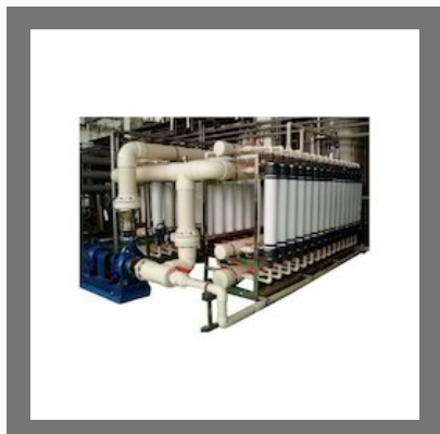
Ultra Filtration Plant
