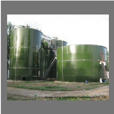
UASB ( Upflow Anaerobic Sludge Blanket Reactor
