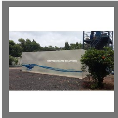
Packaged Effluent Treatment Plant
