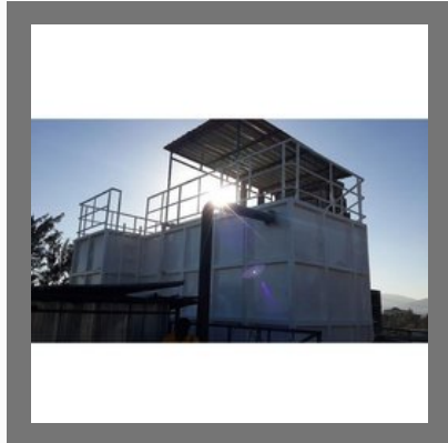
MBBR Sewage Treatment Plant
