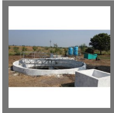
Sewage Treatment Plants
