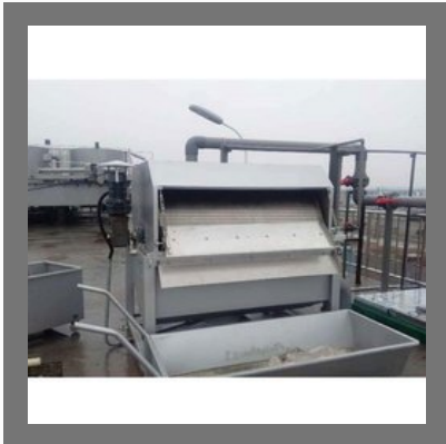
Outward Water Drum Filter
