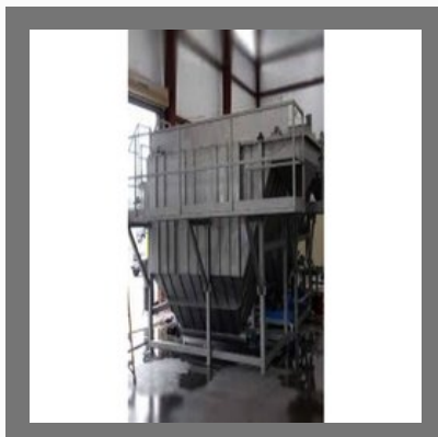
Oil Water Separator
