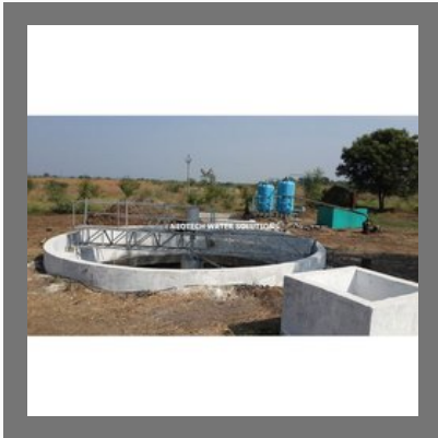
Dairy Effluent Treatment Plant
