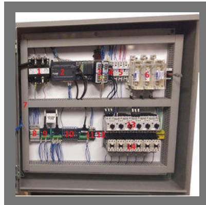
Electric PLC Control Panel
