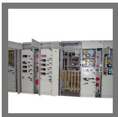
MCC Control Panel
