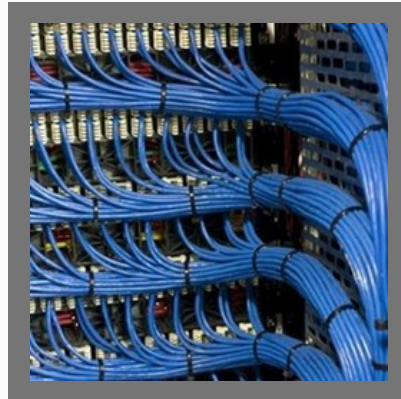
Structured Voice Data Centre Service
