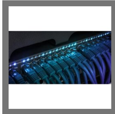
Networking Data Centre Service
