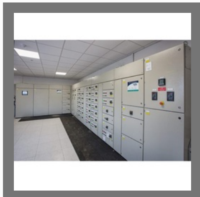
Effluent Treatment Plant Control Panel
