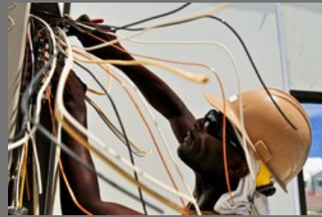
Electrical Maintenance Services
