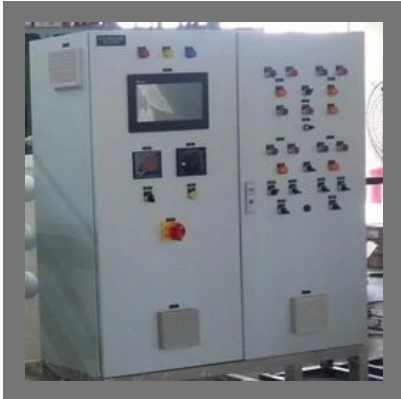
PLC With HMI Control Panel
