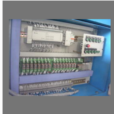
PLC Operated Control Panel
