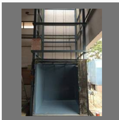
Industrial Passenger Elevator
