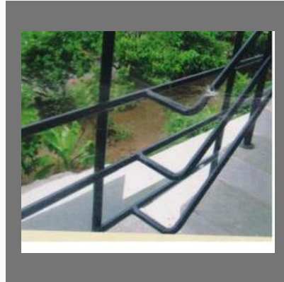
Mild Steel Handrail
