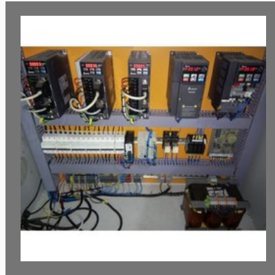
Electric Control Panel
