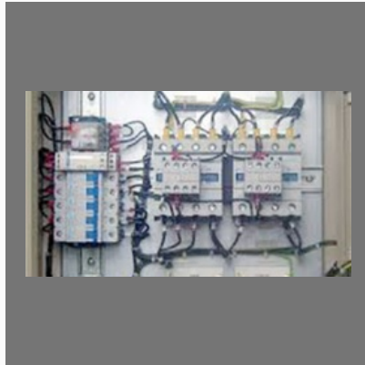
Auto Changeover Panel
