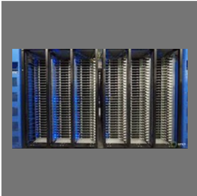
IT Server Rack PDU
