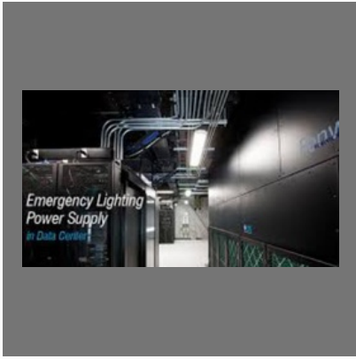
Raw Lighting And Emergency Power DB
