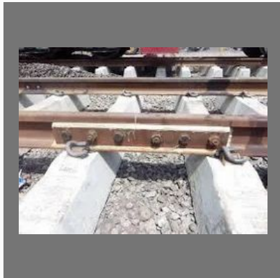
Glued Insulated Rail Joints
