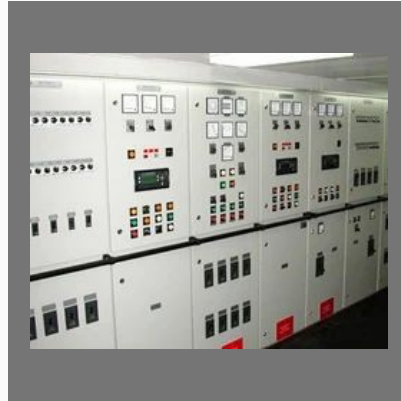
Electrical Control Panel
