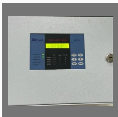
Fire Alarm System
