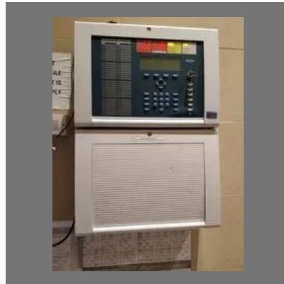
Esser Fire Alarm System
