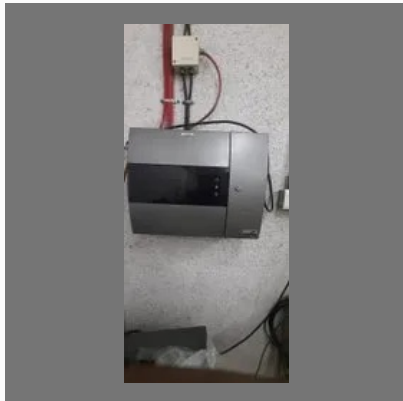
Cooper Fire Alarm System
