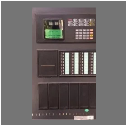
gst fire alarm system
