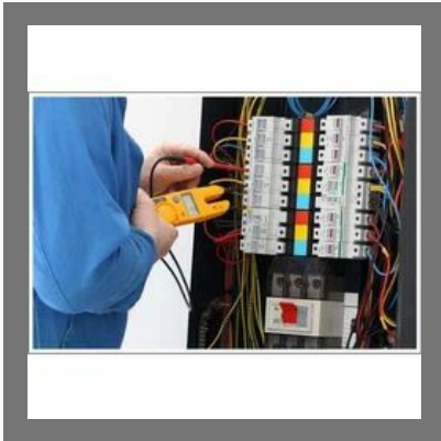
Electrical Contractor Services
