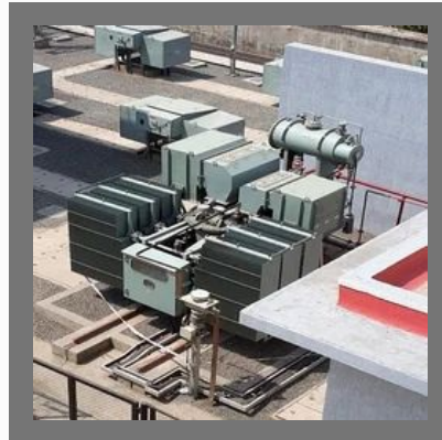
Electrical Transformer Installation Service
