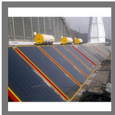
Industrial Solar Water Heater
