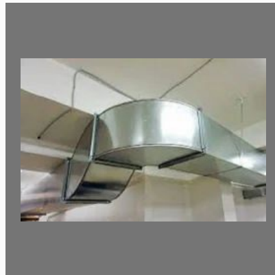
Commercial Kitchen Ventilation
