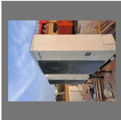
Air Conditioning Hvac System
