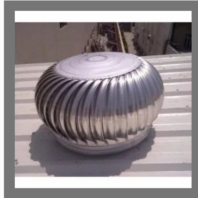
Air Ventilation System
