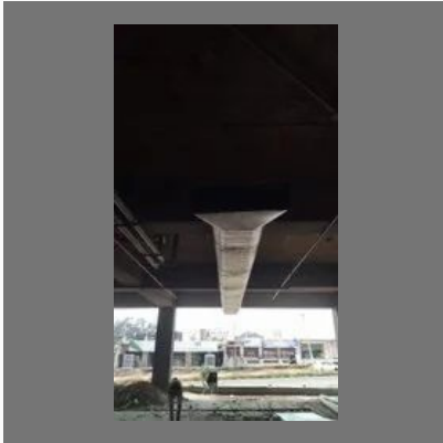
Hvac Ducting Contractor
