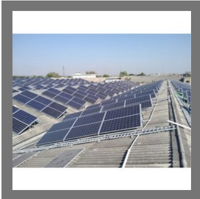
On Grid Solar Power Plant
