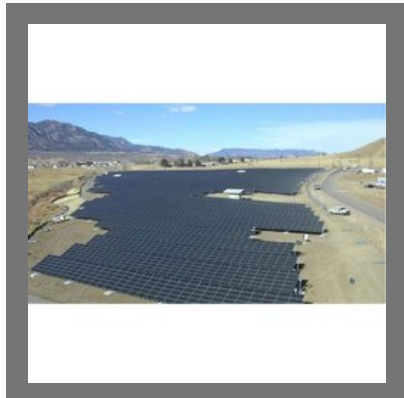
Commercial Solar Power Plant
