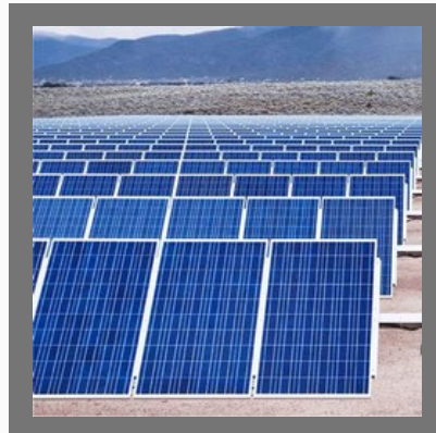
EPC Solar Power Plant
