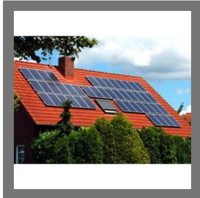
Domestic Solar Power Plant
