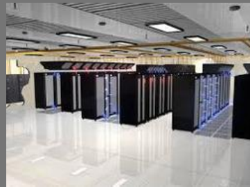
Data Center Solutions
