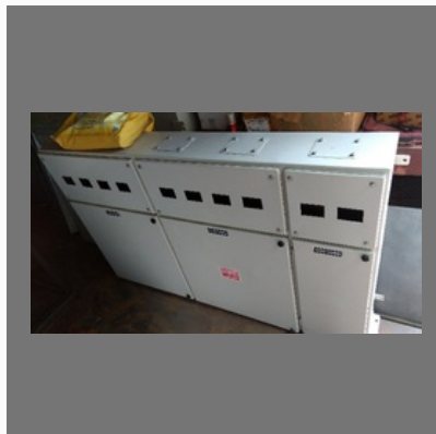
Electric Control Panel
