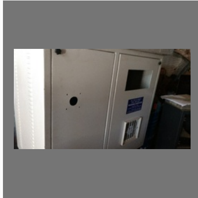
Solar Control Panel
