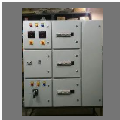
Electric Control Panel Petrol Pump Application
