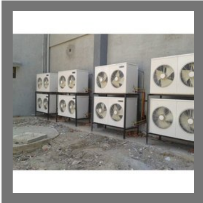
Central Air Conditioning System
