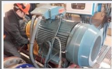
Modification of equipment for Provisions for PM & CM
