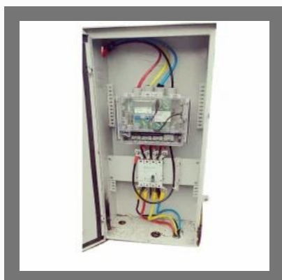
Power Distribution Box
