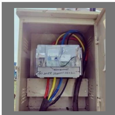
Industrial Electrical Sub Meters
