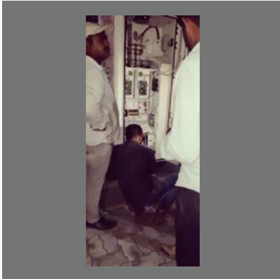
Electric Control Panel Installation Service
