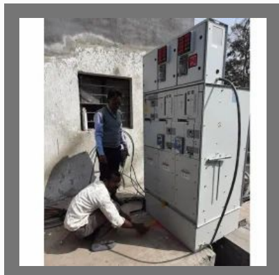
Distribution Box Installation Service
