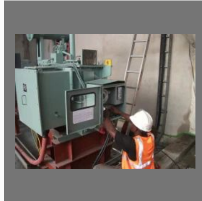
Electrical Transformer Installation Service
