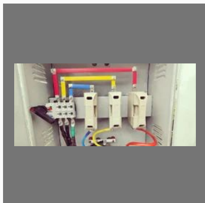
Electrical Fuse Box
