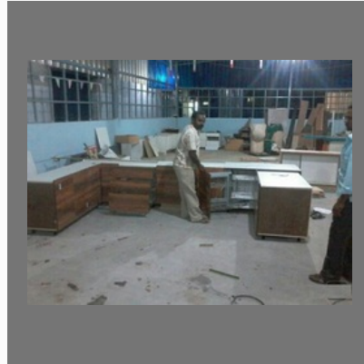
Kitchen interior services
