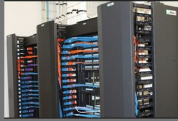
Structured Cabling Service
