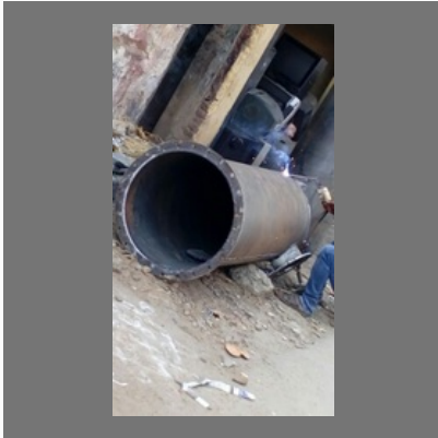
Industrial Water Plant
