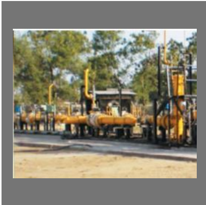
Gas Pressure Reducing Et Metering Skids
