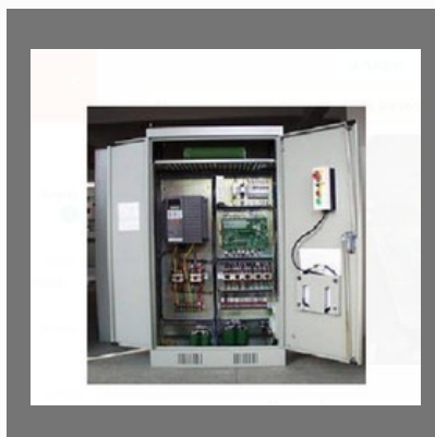
Elevator Control Panel System
