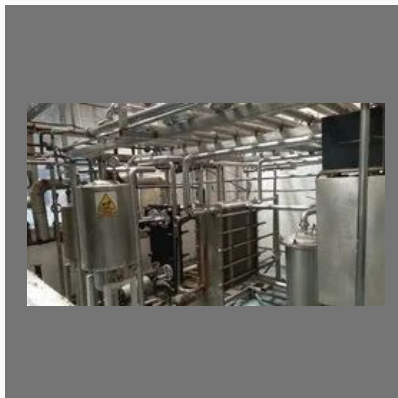
Polyester Plant /Modular Process Plants
