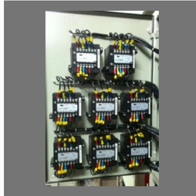
Industrial Switch Board
