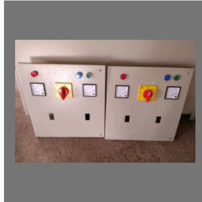
Electrical Control Panel
