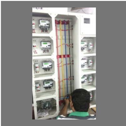
Electric Control Panel
