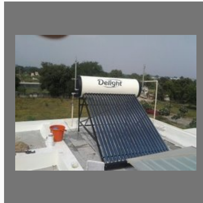
Solar Water Heater
