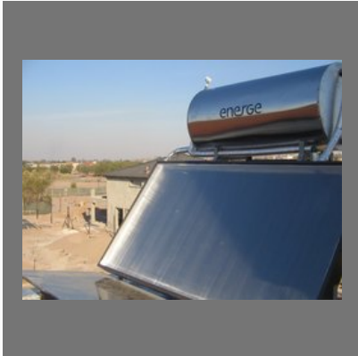
Solar Water Heating System
